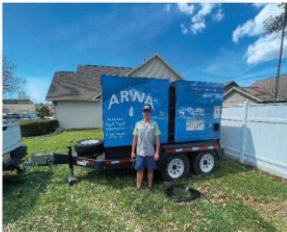
ARWA Generator being delivered to Englewood
