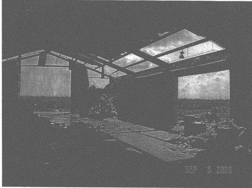
USDA Research Farm Equipment Maintenance Facility Damage
